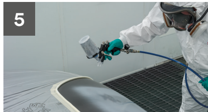
5 Apply high build primer to repair area using 3M™ Accuspray™ Gun and 1.8mm nozzle.
