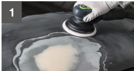
1 Key around the repair area using 3M™ abrasive discs, grade P320 and P500.
